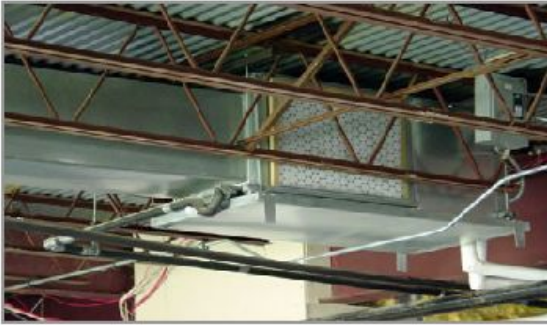
High-Efficiency Commercial Geothermal Heat Pump – Above Ceiling Installation
